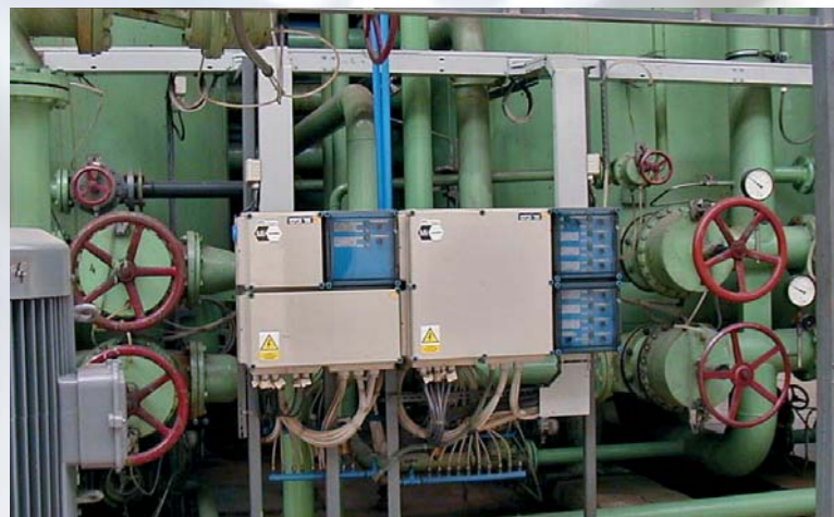
Mi distribution board in the chemical industry
