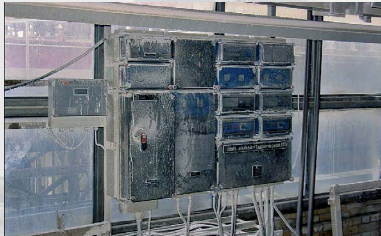
The distribution boards in a zinc mining company are exposed to extreme amounts of dust and dirt.
