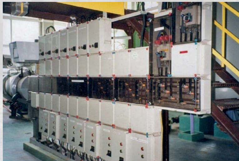
General power supply for keeping production processes up and running in a mine in combination with a generator.
