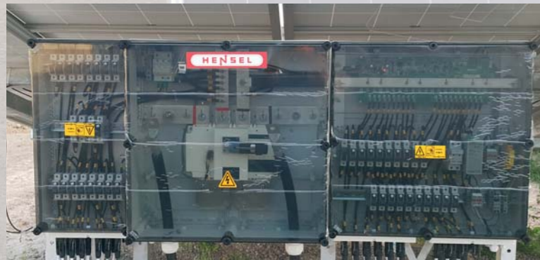
Individual product solutions with integrated string monitoring for a large PV plant ensure the reliable distribution of electricity in Thailand.
