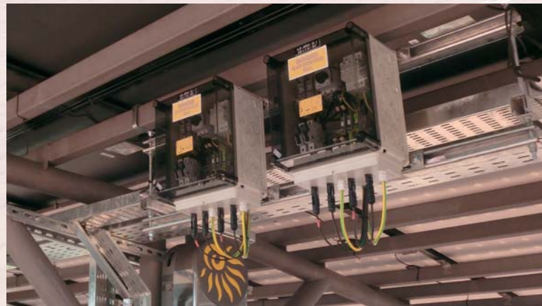
Numerous Hensel PV generator junction boxes ensure a reliable distribution of generated PV electricity.
