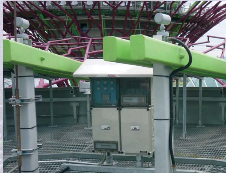
PV power inverter collectors are installed on the Supertrees in Singapore.
