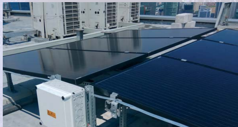
Numerous PV generator junction boxes are installed on the roof of the Marina Bay Sands Hotel.
