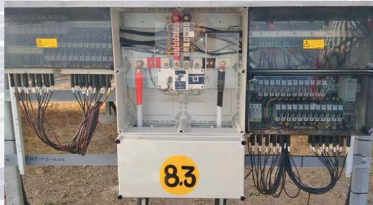
PV distribution boards after the expansion of a PV plant in Chennai, India.
