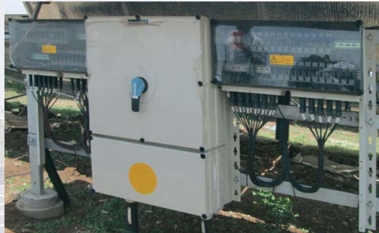
PV distribution boards before the expansion of a plant in Chennai, India.
