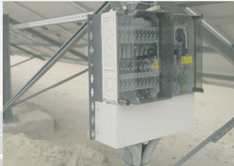
PV distribution boards close to a water source in the desert for a network-independent water pump system
