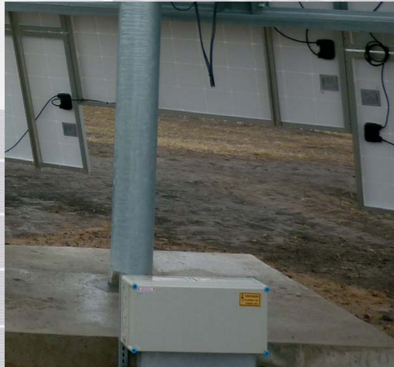
Numerous solar trackers in a solar park in Újszilvás (Hungary) generate 635,000 kWh a year. The power inverters were connected using individual Hensel product solutions.
