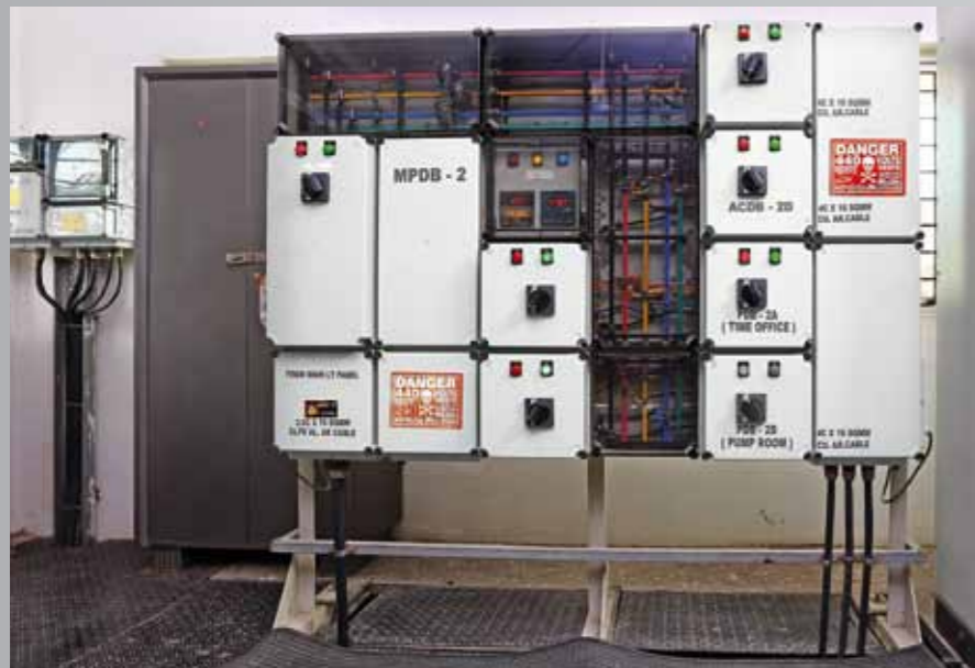
Main power distribution board installed at a foundry
