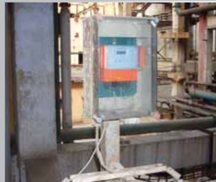
Instrument enclosure at a pumping station
