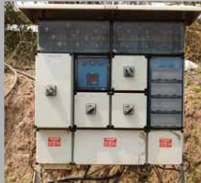
Sub distribution board installed at a hydro electric plant.
