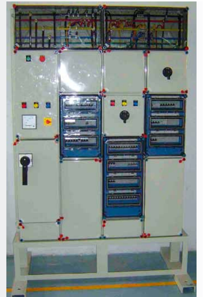
Main power distribution board for a petrol station
