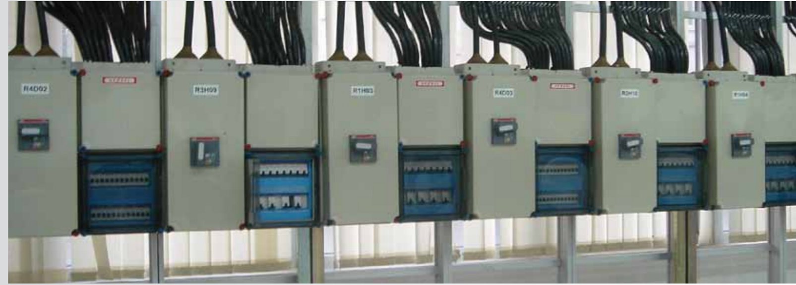
Lighting control distribution boards in use at a mobile phone manufacturing plant
