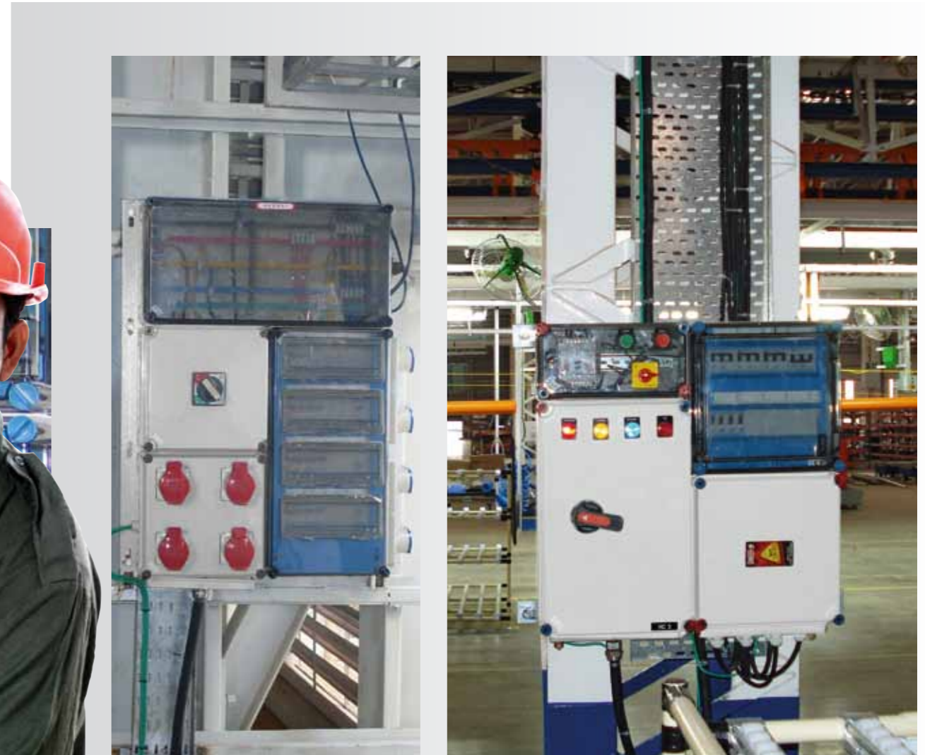
Shop floor distribution board with CEE sockets installed in an engineering fabrication plant.
